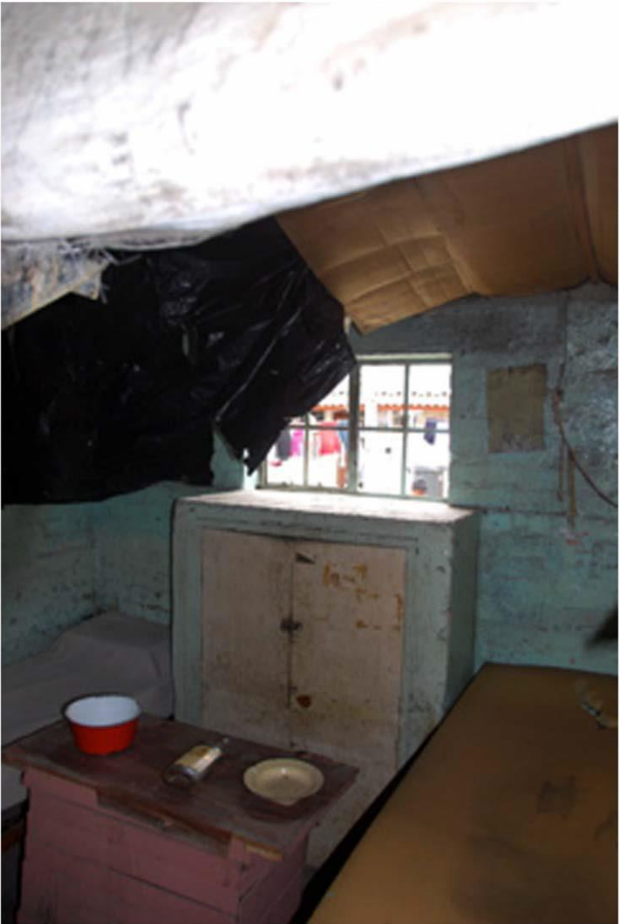
Figure 10. Sagging ceilings, March 2010. Deterioration of makeshift interiors posed questions of removal, replacement or rehabilitation and re-securing of the original material. Copyright, William Martinson.
